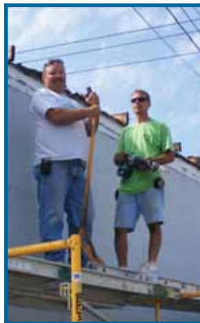
Bruce Rookstool and his foreman, Gary Onslager, replace a roof this summer at RP Auto in Huron.
